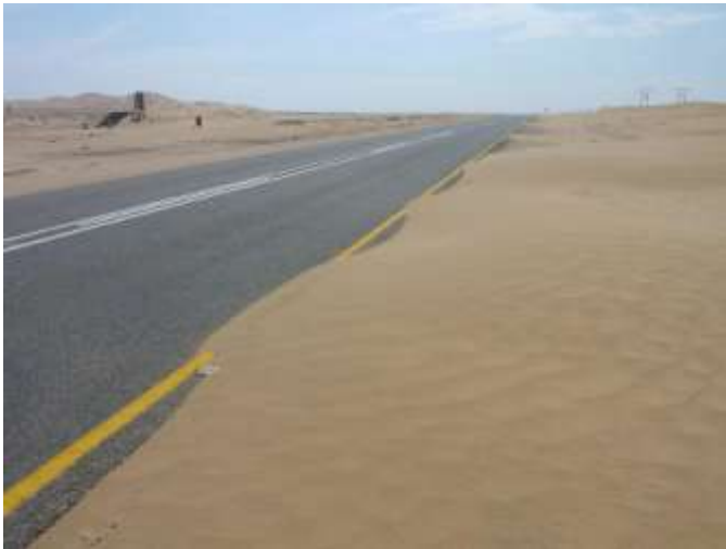
Figure 12. Sand encroachment on the C14 road. Photo by Mattias Bovin (2010)
